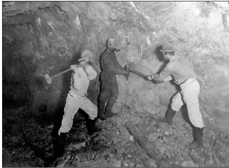
Two handed jacking like this looked and sounded impressive, but the resulting saving in time and money were insufficient to make it a common practice.
