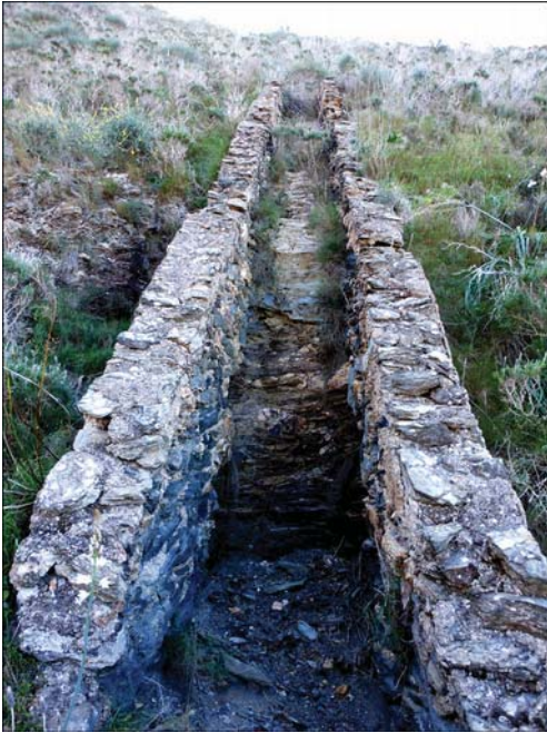
One of the channels used to collect water on the hillside. These used to be covered.
